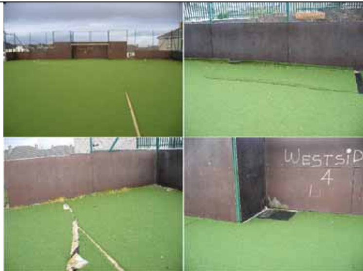
Fig. 11. Things to look out for (before they ever get like this) (Top left) seam failure. (Top right) poorly patched areas. (Bottom left) in-laid line failure. (Bottom right) graffiti. Get rid of graffiti quickly otherwise it encourages more.
